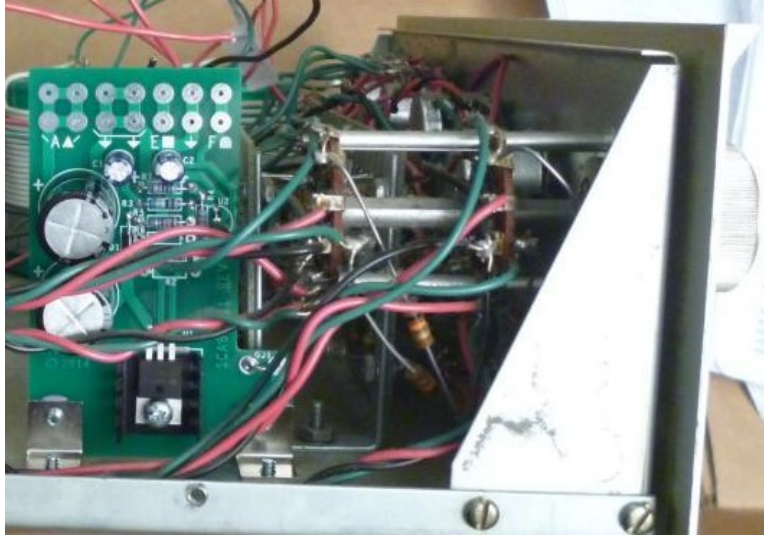
Figure 8-New Power Supply Installed in SCA80(Q)
