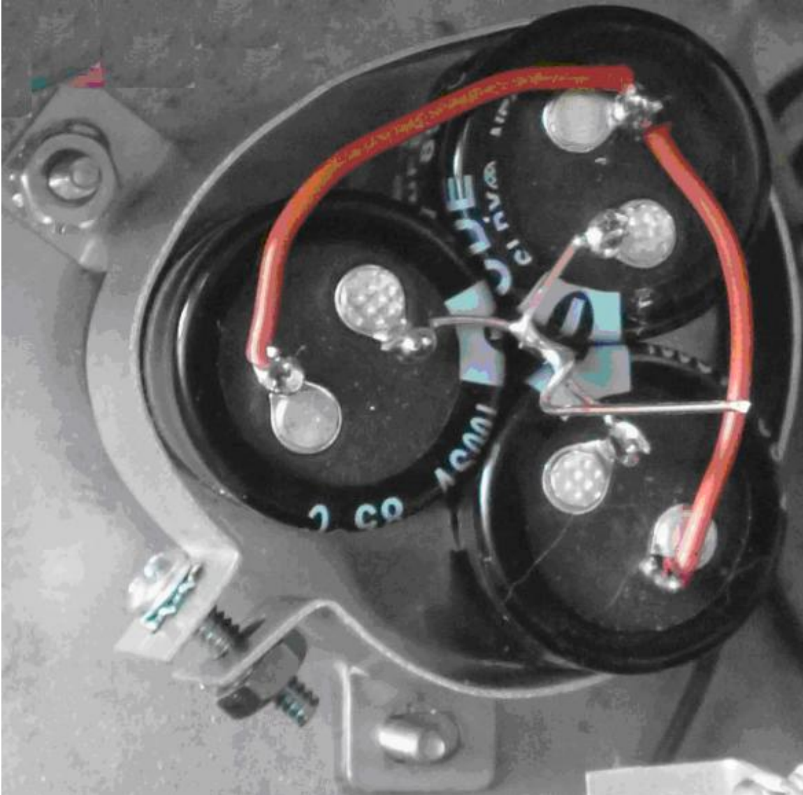
Figure 4-Soldering the ground and positive harnesses on the new C9 dynamite capacitor arrangement
