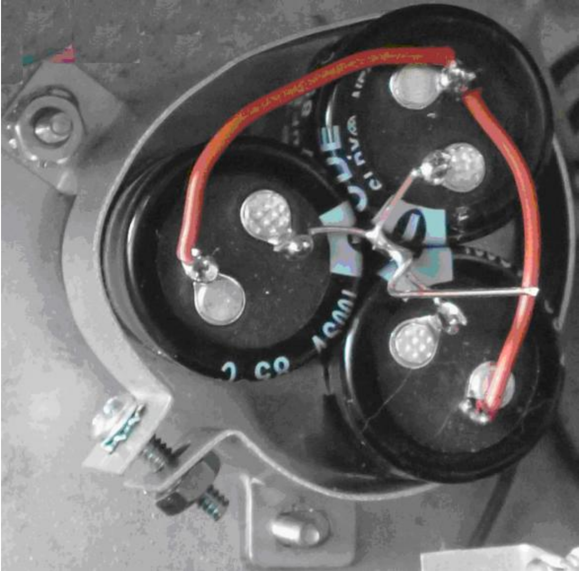
Figure 5-Soldering the ground and positive harnesses on the new C9 dynamite capacitor arrangement
